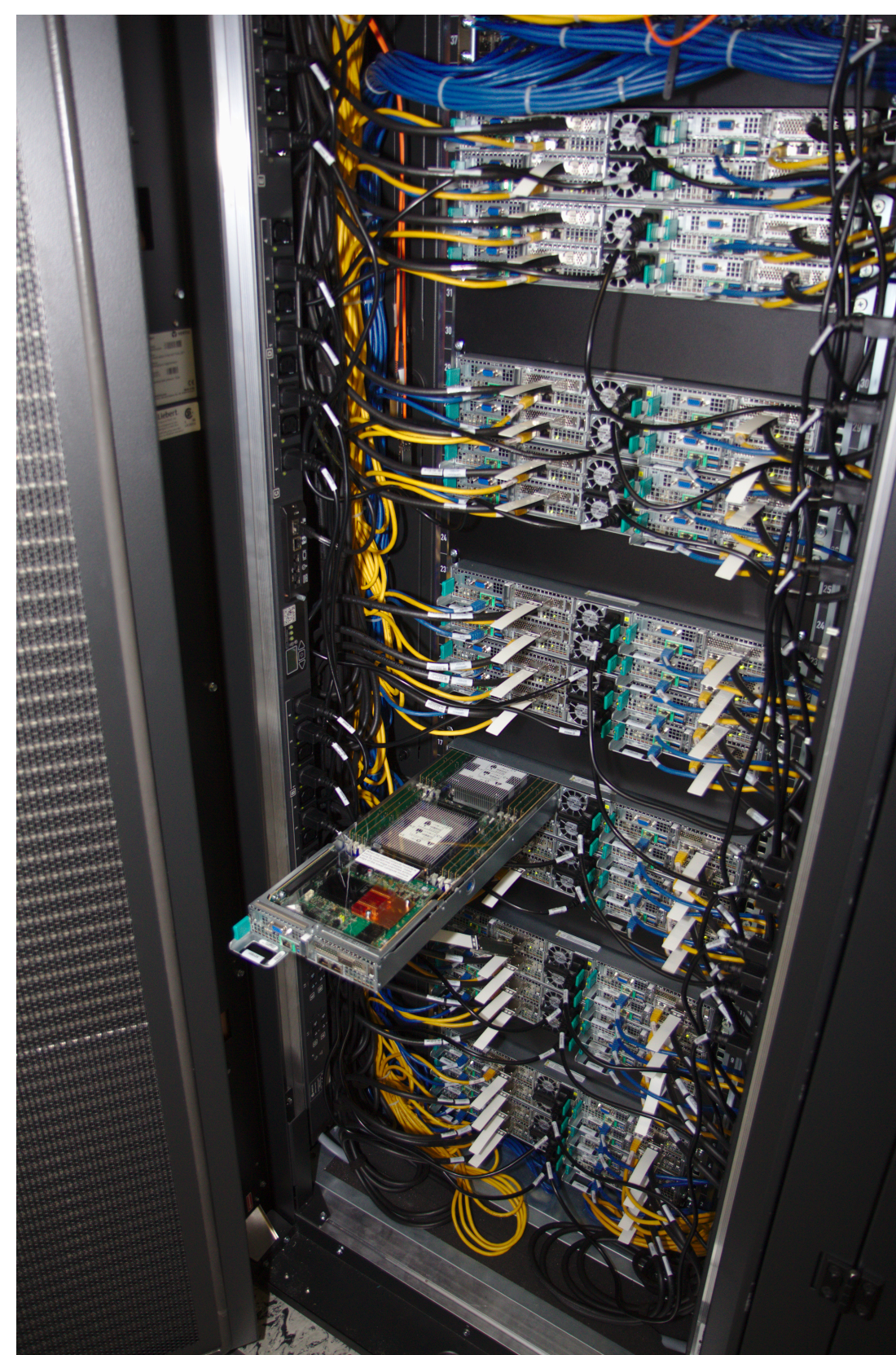
Figure 2: Open backside of rack 8.
