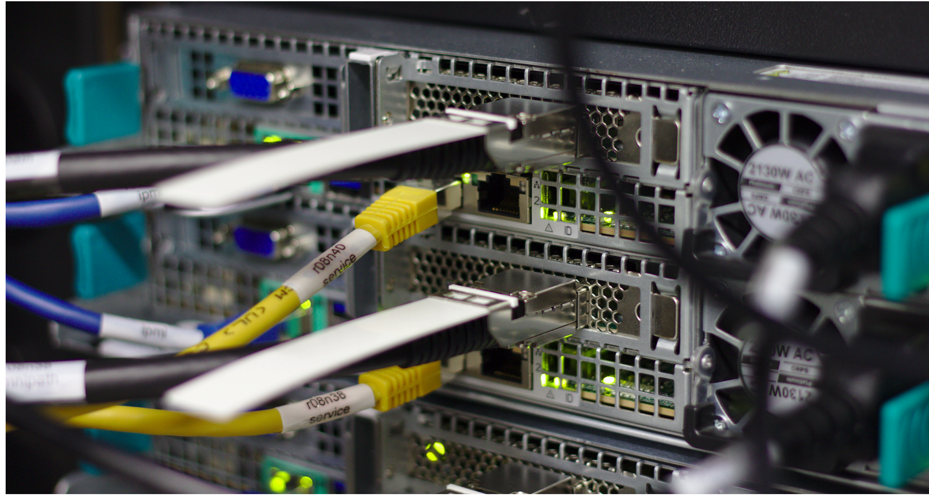
Figure 1: Ethernet and Omni-Path connections at the backside of node 38 and 40 inside rack 8.
